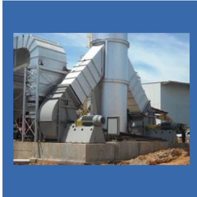
Smoke Spill Unit
