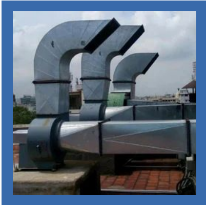
Air Ventilation System
