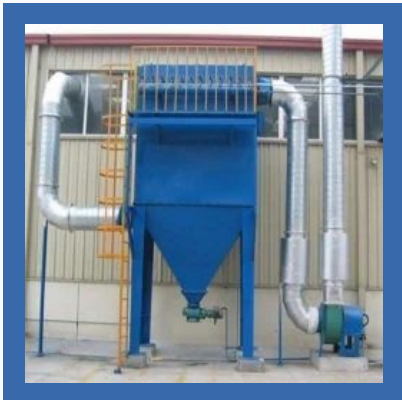
Dust Collector System
