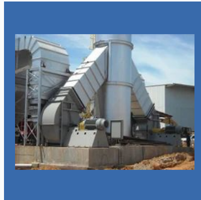
Smoke Exhaust System
