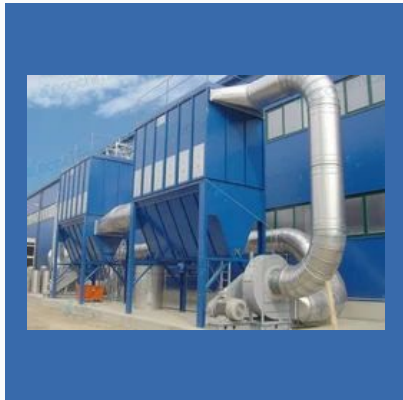
Pollution Control Device
