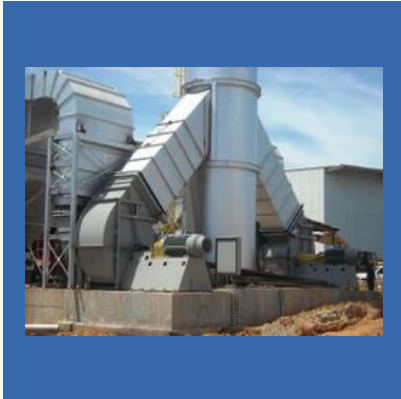
Fume Extraction System
