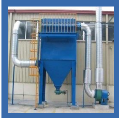
Dust Collection System
