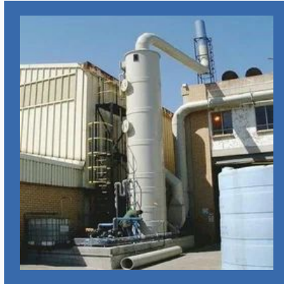
Packed Bed Scrubber
